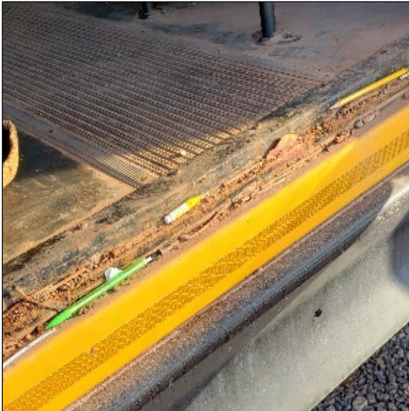
Stuck Emergency Door a Safety Hazard
